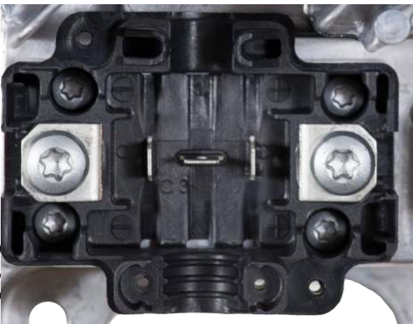
Close-up view of battery temperature sense and interlock blade terminals within the IC650's DC output block.
